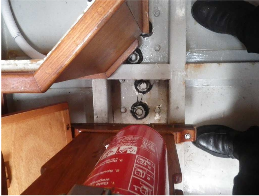
Figure 8 - Nuts and threaded rods and bolts that hold the keel in place seen from inside the sy CAPELLA
